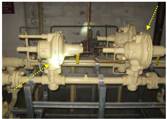
Photograph 18. Loading Dock level S: Gas Meter room – Gas pump-set with modern diaphragm gaskets.
